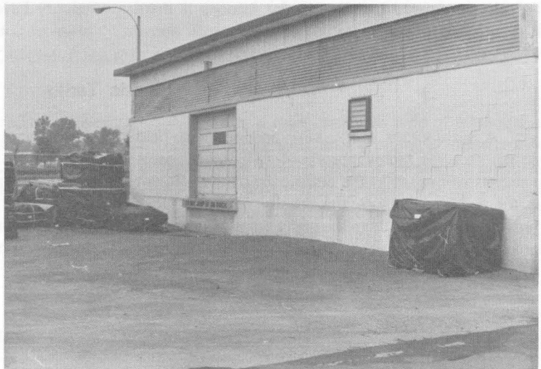
Figure 11. Pre-construction foundation studies can aid in preventing extensive cracking in masonry walls and concrete foundations such as those shown here.
