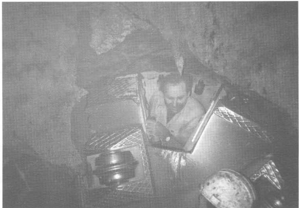
Figure 8. Low-gravity oil seeping through shale bedrock during construction of Trans-Missouri River Tunnel.
